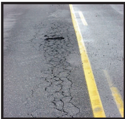
Figure 3.15.3d – Surface begins to pothole and rut.
