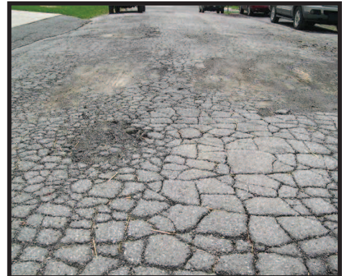
Figure 3.15.3g – Whole road surface needs replaced.
