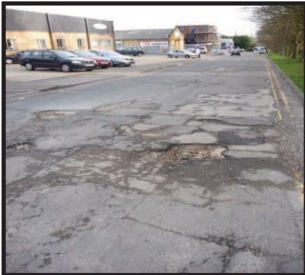
Figure 3.15.3f – Defects become more widespread.
